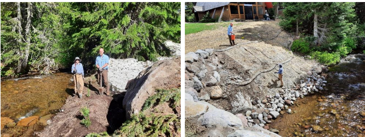
SCA interns Beth Anderson (left, left photo) and Dan Fawcett Jr. (right, left photo) plants western red cedar and willow stakes along a new culvert in Camp Creek at West Ski Bowl.
